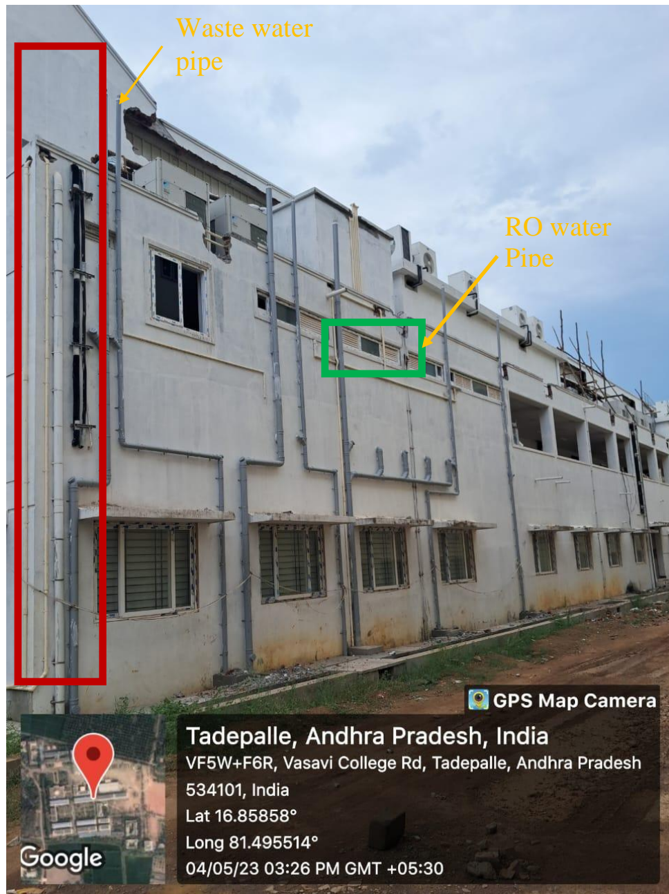
Fig. Water distribution pipes in Auditorium block
