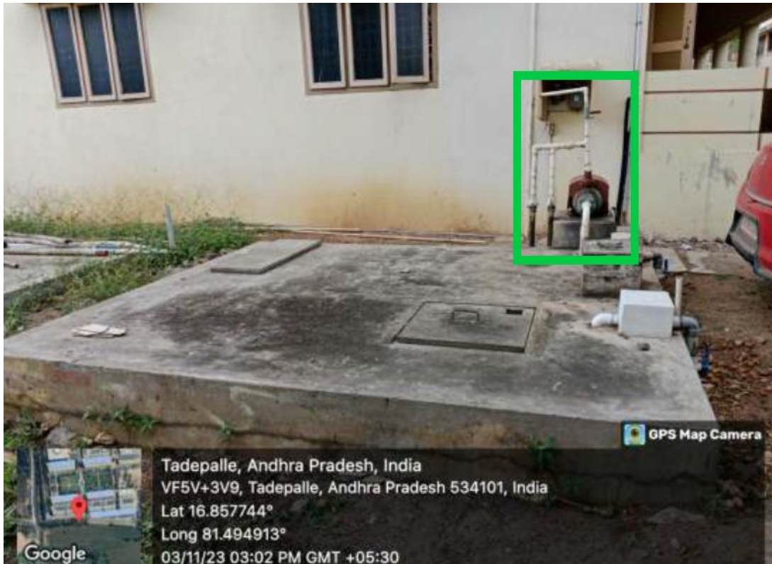
Fig. The sump with two 3HP motors located near CSE Block-2 is used to supply the RO Waste water to CSE Block-2, Mechanical, Civil and MBA block wash areas.
