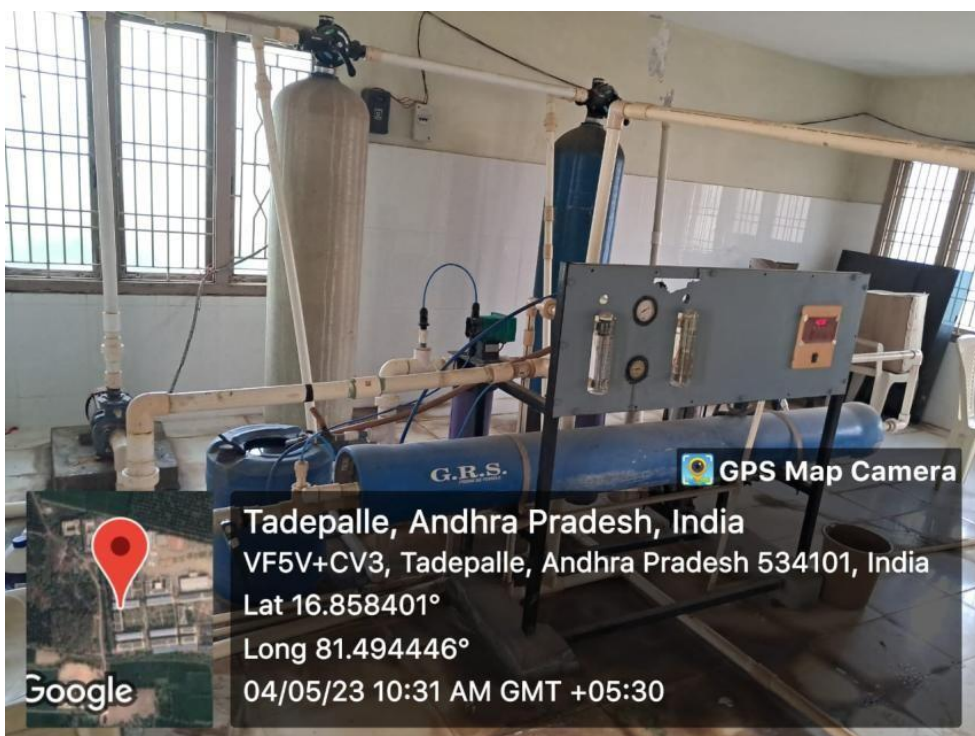
Fig.RO Plant at ECE Block, SVEC
