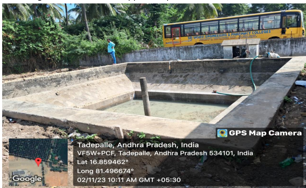
Fig. Water tank with 50000 liters capacity
