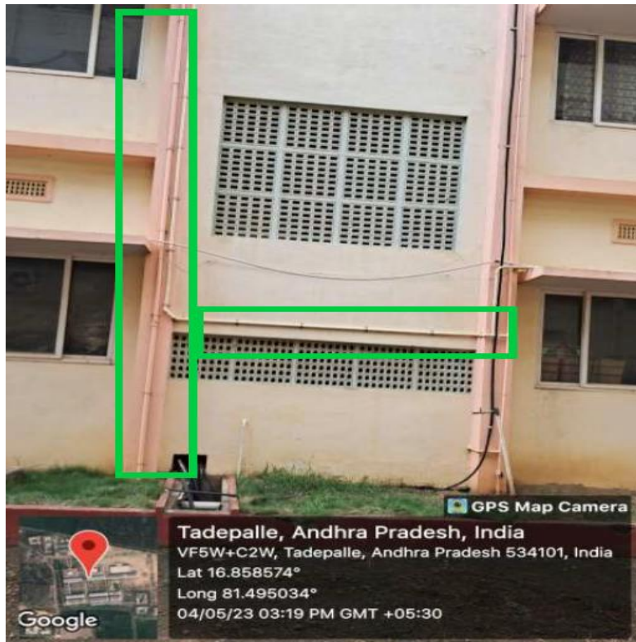
Fig. RO water distribution pipes at ECE block
