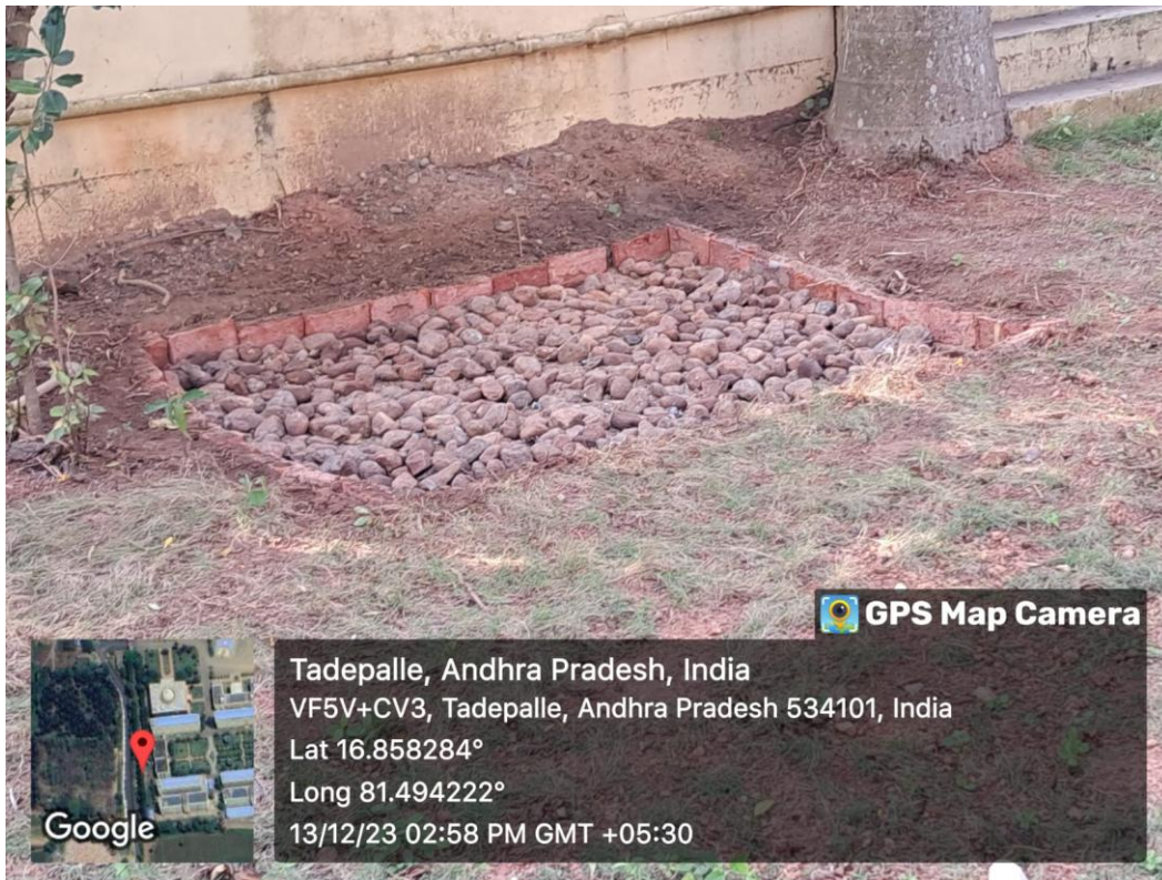
Fig. Rain water harvesting pit-3 (At the Backside of ECE Block-1)
