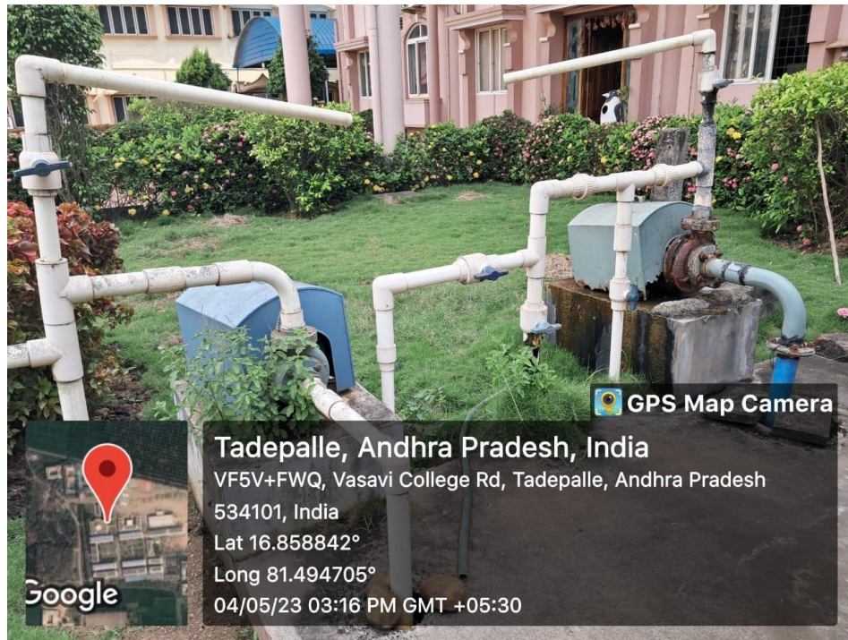
Fig. Bore well water saved in tank and supplied to ECE Block-2(D block) -RO unit for purification
