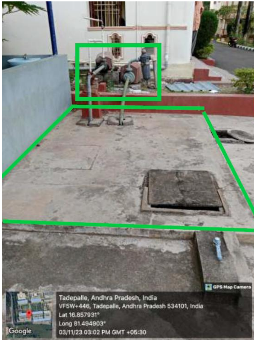
Fig. The sump with two 3HP motors is used to supply (RO waste water) to ECE, EEE and CSE block-1 wash areas.
