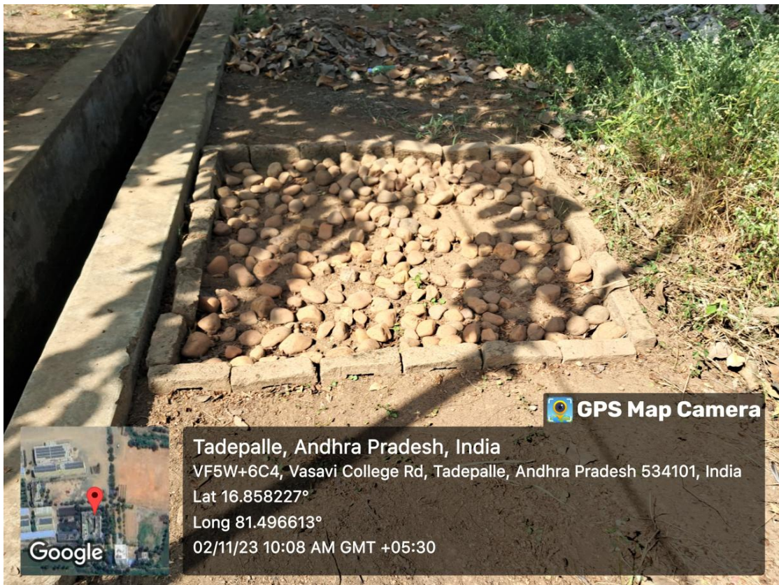
Fig. Borewell/Ground water recharging through Rain water harvesting pit-2( near Ladies hostel)
