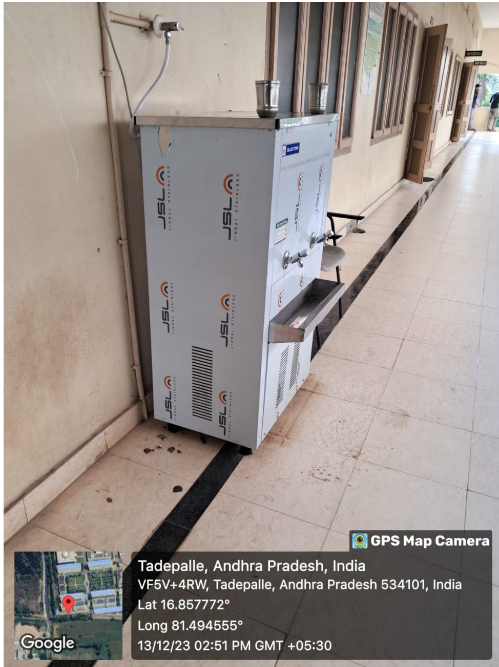
Fig. Drinking water point at BSH block (First floor)
