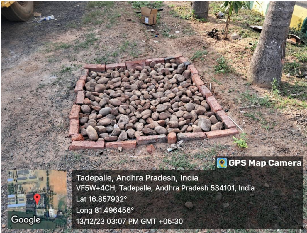
Fig. Rain water harvesting pit-4 (Opposite to BSH Block)
