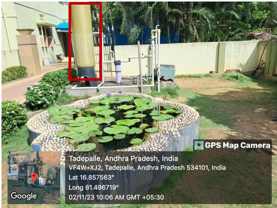
Fig. Bore water filter for supplying water to Ladies Hostels
